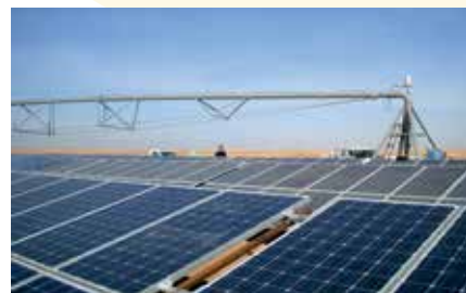
PV Array at Pivot Center
