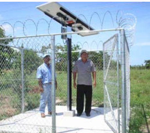
Effective theft protection: Panel and tracker fenced in and protected by barbed wire
